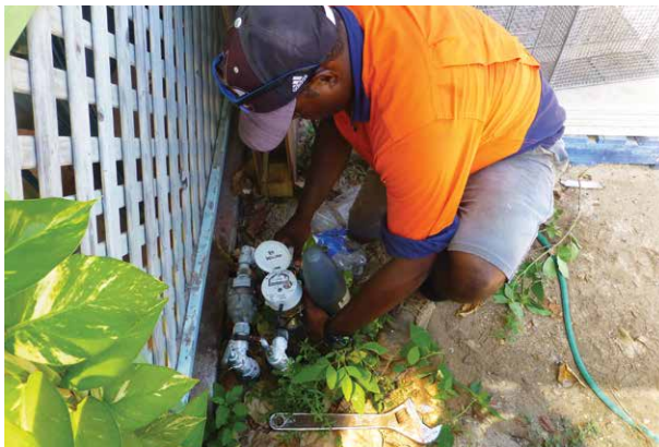
Figure 16. Installing smart water meters. (Source: M. Jackson. Photo used with permission from participant)
