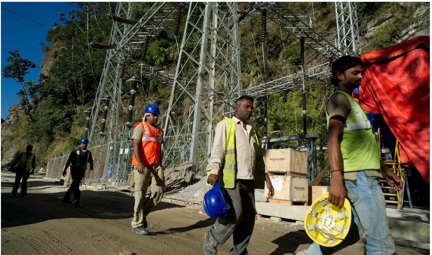
Green Power Development Project in Bhutan (ADB).
