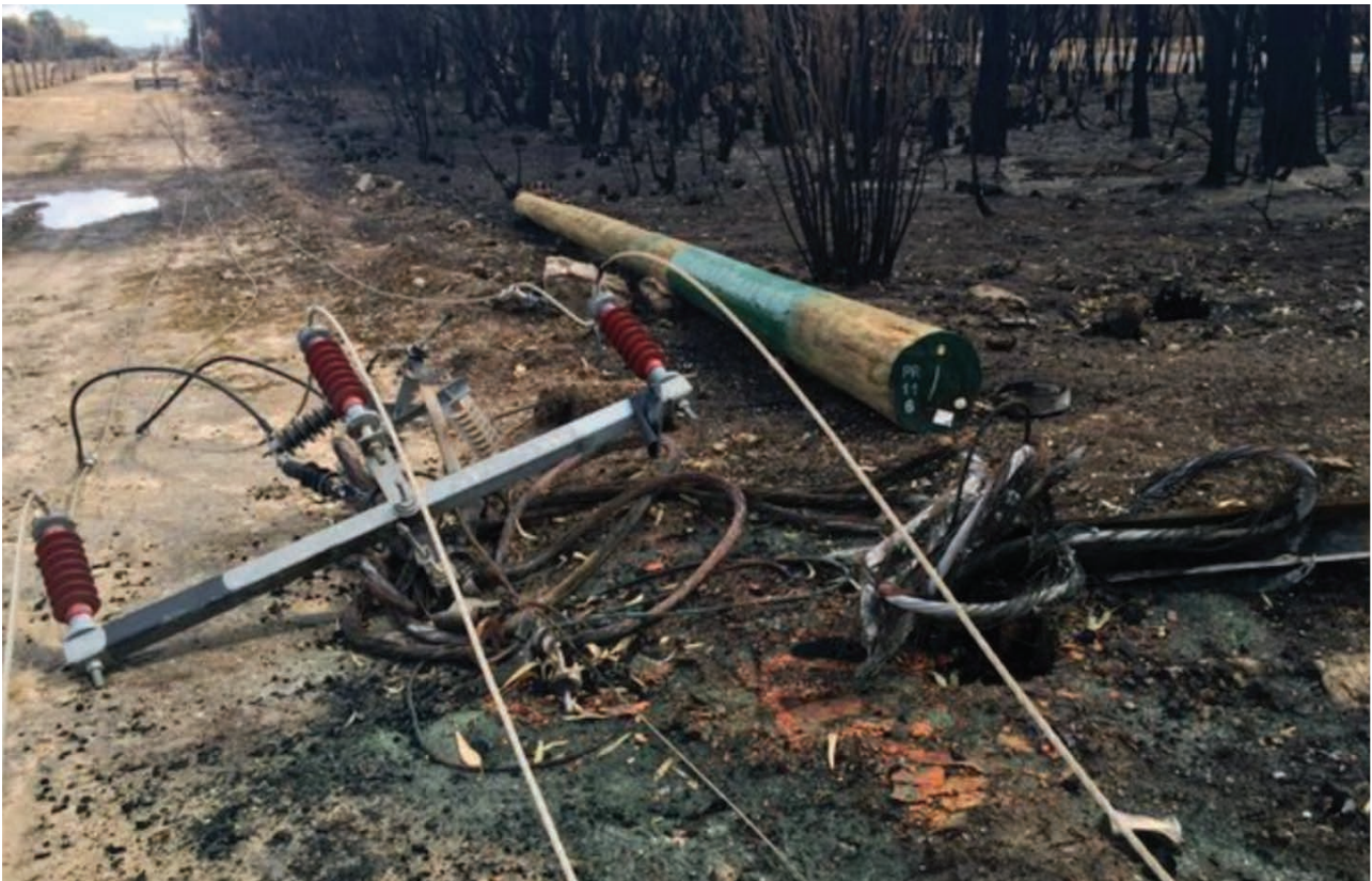
Image 12: Loss of power infrastructure from the Australian bushfires, 2019–2020
